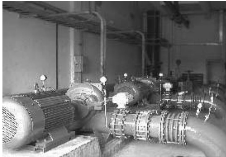
Figure 4: New Pumping Systems
